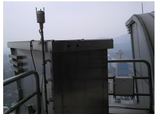
Fig 3. Photo of the instruments at 34 th floor of Taipei 101 Tower
